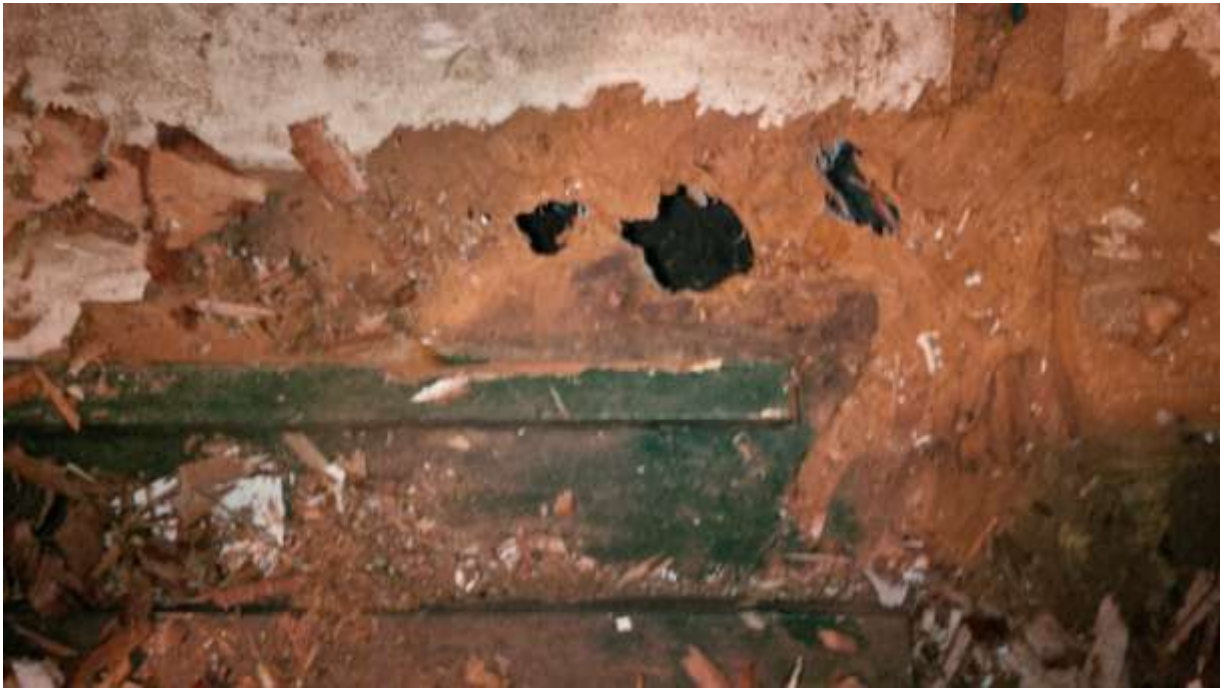
Fig 1a: Dry Rot
