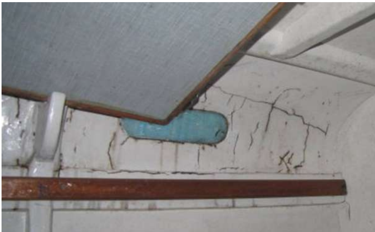
Fig 2: GRP repairs to be removed
