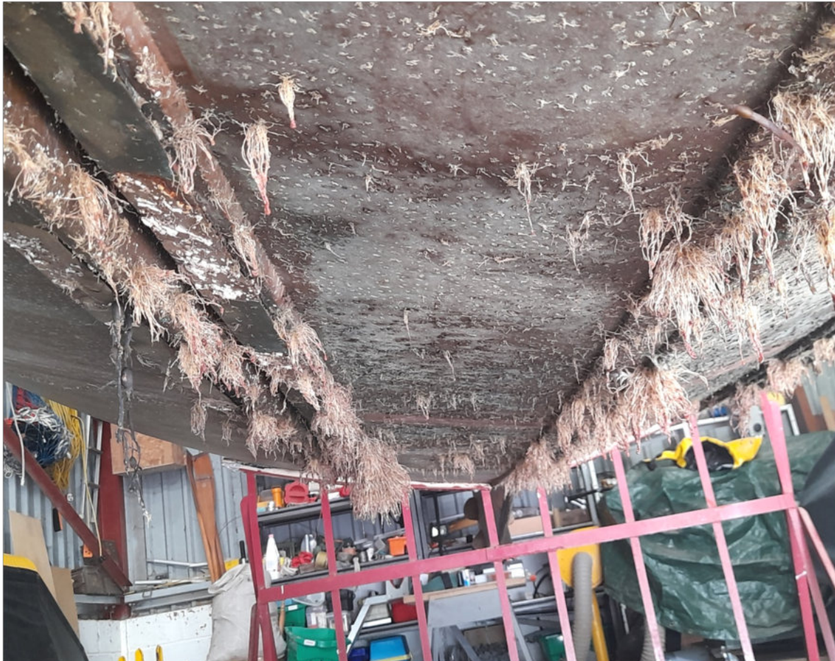
The bilge area after pressure washing with weed still attached that could only be removed by scrubbing with a course Scotchbright pad
