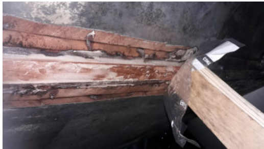
Groove routed out, screw holes plugged with dowels and new batten epoxied in place
