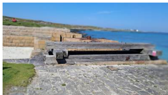
Stop Logs to protect the harbour from storm waves but all now unused. Note the grooves in the harbour walls beyond.
